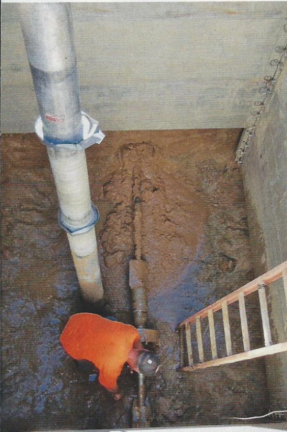
As another bore is completed, Trenchless Flowline employee Kelly Lindeman prepares the drill rods for pipe pullback. Photos: Trenchless Flowline
