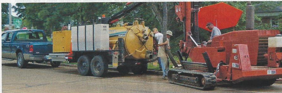
Bore slurry was removed from sight relief holes during pullback by a trailer-mounted Vac-Tron MC855 SDT sewer jetter.
